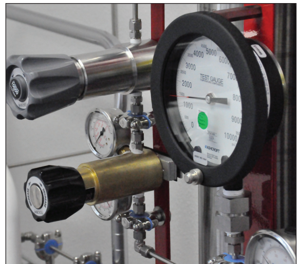
Gauge for High-Pressure Accumulator Tank Used During Calibration
