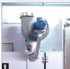
8 Air change and cooling extractor
